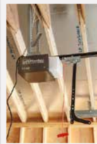
Garage Door Opener
